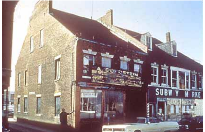
Photograph from the 1970s of 17–23 Front Street showing its condition prior to restoration. The granite store front system is missing and some of the second floor windows have been replaced by a picture window. The splayed lintels on the remaining windows and the surviving dormers served as models for the reconstruction of the missing features. Courtesy of William Tinti.
