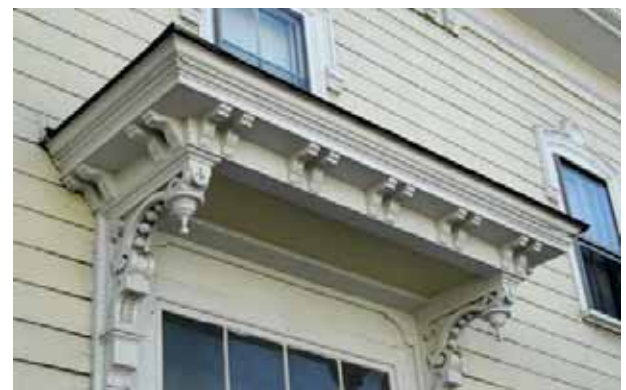
Original details such as this elaborate Victorian entry canopy remain on many Bridge Street buildings and should be preserved.
