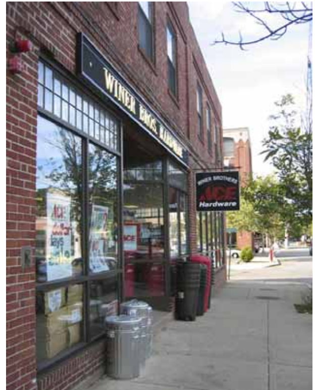
New window systems can be installed that respect traditions of storefront design-note the transom glazing.
