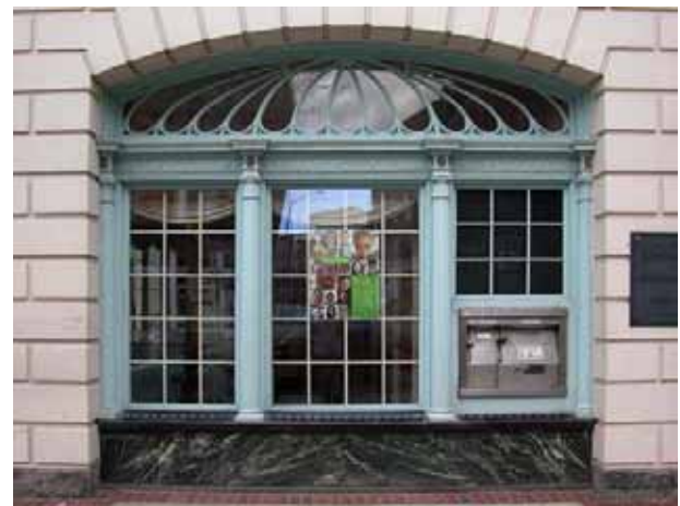
An original c. 1920 storefront with an elaborate curved transom on Washington Street. Typical of Salem's more substantial early twentieth century commercial buildings, this is in the Colonial Revival style with traces of Art Deco.
