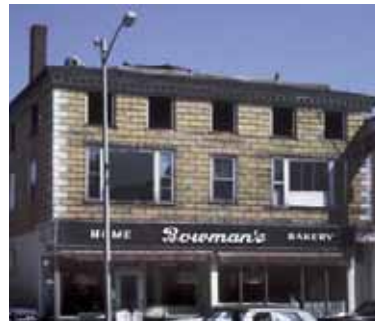
Removal of artificial siding reveals the original rusticated board siding and the original window placement of the upper stories. Courtesy of City of Salem.
