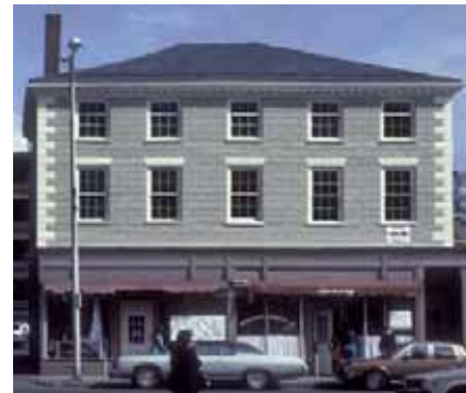
Restoration of the upper stories as completed in 1983 with 6/6 windows based on historic photographs of the building. See page 13 for a photograph of a recently completed rehabilitation of the storefront section. Courtesy of City of Salem.
