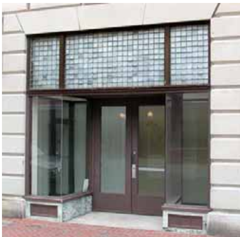
An original c. 1920 storefront with a prism glass transom on the Masonic Building on Washington Street. Several other storefronts with prism glass and copper framing remain in Salem.
