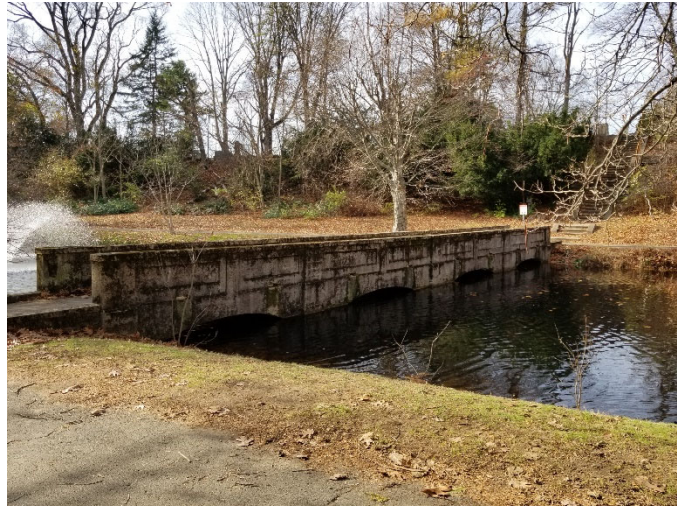
Build up of debris under the Dickson Bridge deck has resulted in spalling, cracking and delamination of the concrete.
