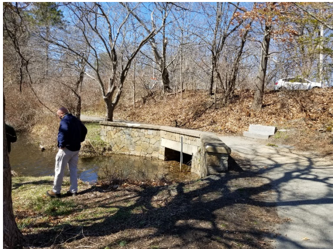
Build up of debris in the culvert at the north end of Sargent Pond has led to failure of the culvert headwall.
