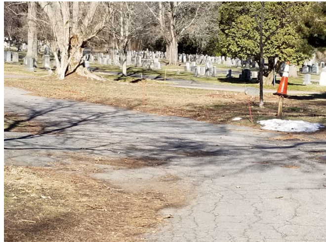
Bituminous pavement throughout the cemetery shows signs of water build up resulting and cracks and failure.
