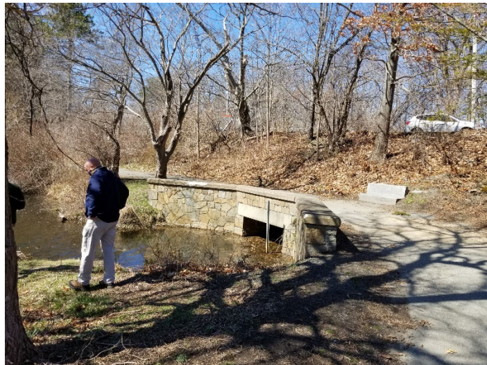
Phase 2 involved assessing the condition of the ponds and historic structures, including the culvert at the north end.
