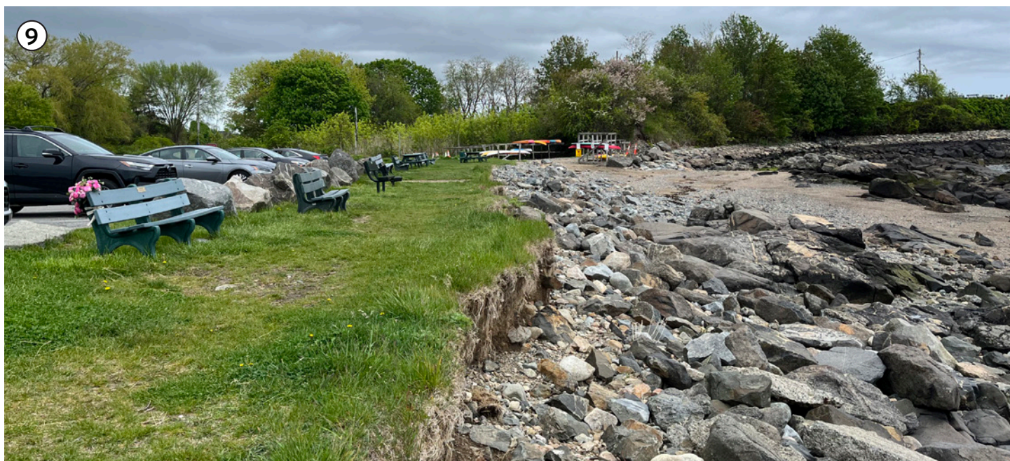
FIGURE 9: THE STEEPLY ERODED EDGE OF THE COASTAL BANK
