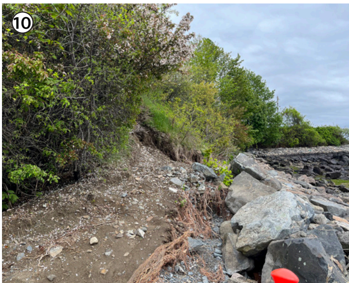
FIGURE 10: BASE OF ERODED PATHWAY
