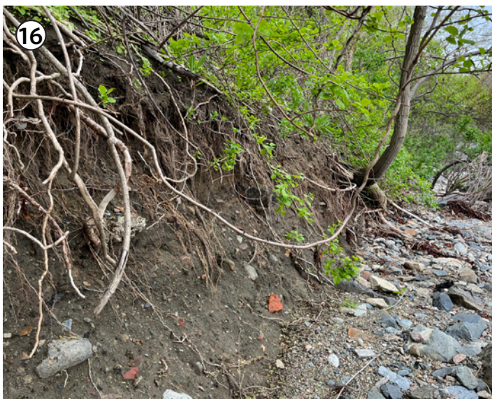
FIGURE 16: ERODED CHANNEL ON THE COASTAL BANK
