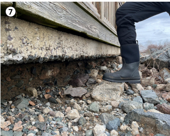
FIGURE 7: SOUTHWEST CORNER OF THE GAZEBO HAS BECOME UNDERMINED
